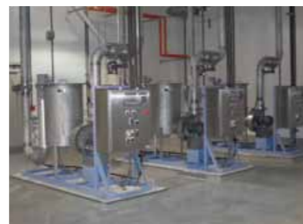
Ozone Destruct Unit
